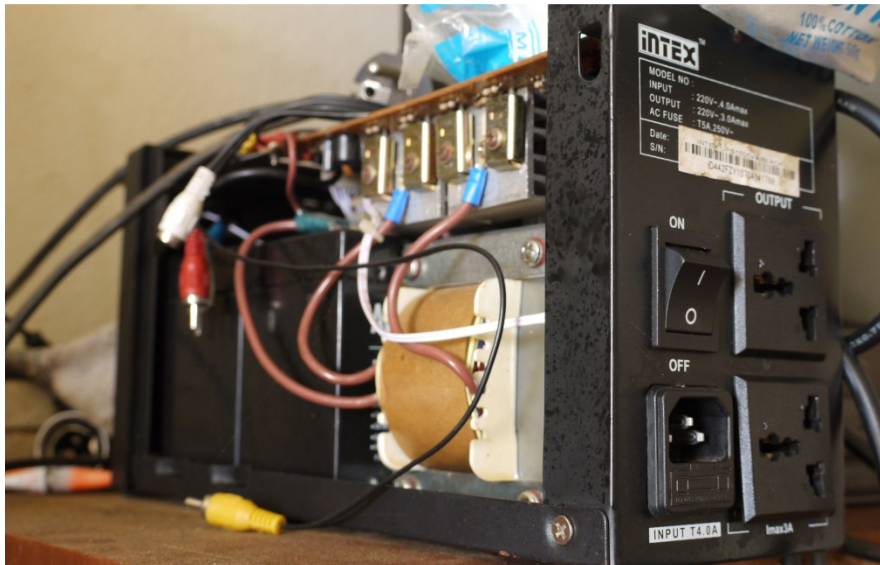
Fig. 6.3 Small uninterruptible power supplies are frequently used to provide emergency power to a load when the main electricity fails. Many of them are damaged by electrical surges.
