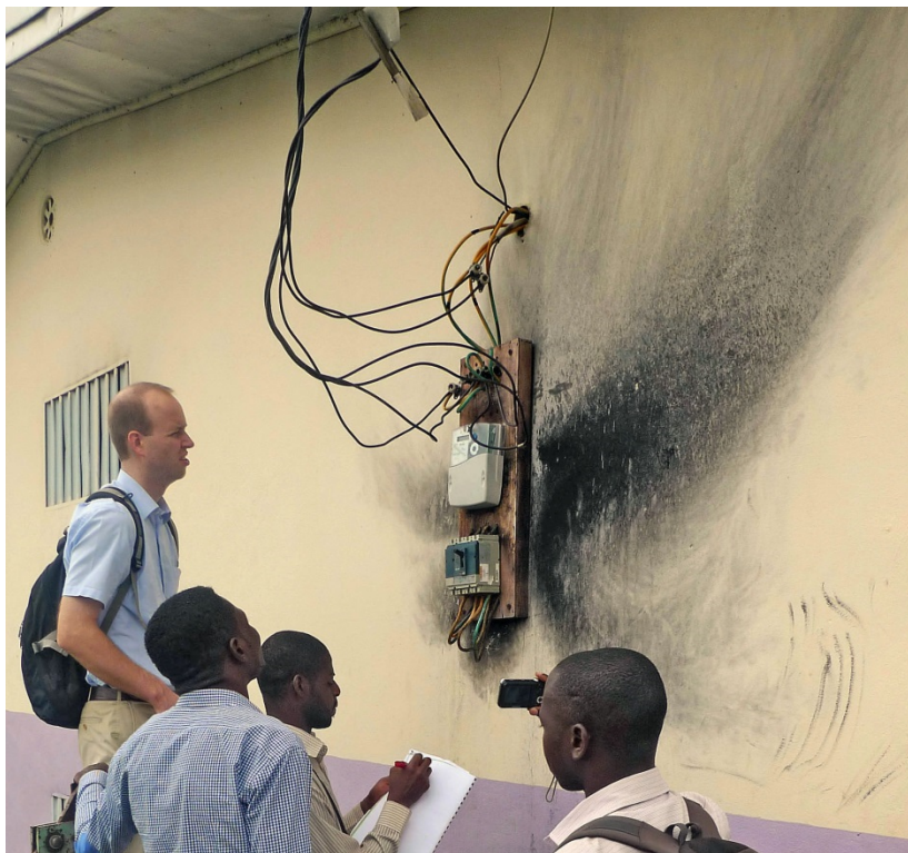
Fig. 6.2 Marks of fire on an electric panel exposed to weathering
